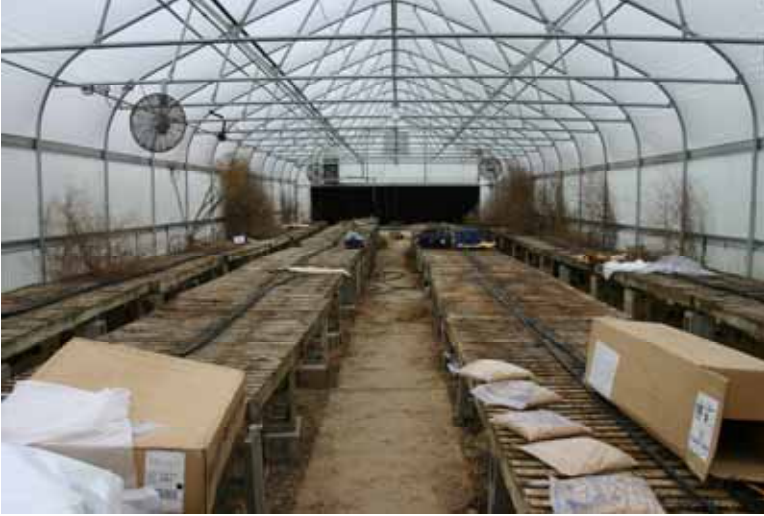
Photo 5. The degraded aquatics greenhouse shortly after acquisition.
