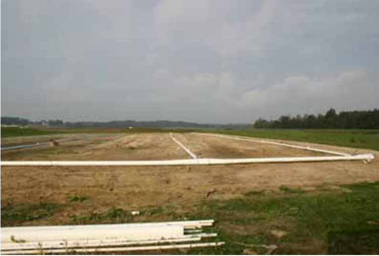
Photo 3. The initial phases of construction, the gravel pad and installation of the PVC water and air lines.
