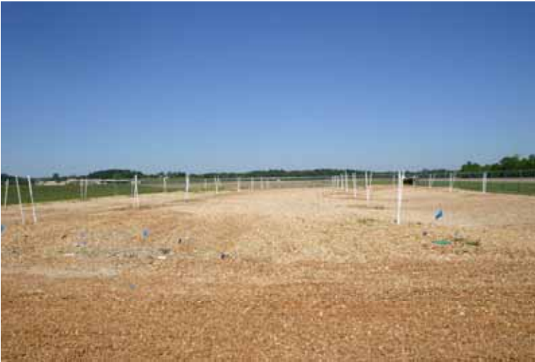
Photo 4. Water and air lines stubbed up out of the ground to supply water to experimental tanks.
